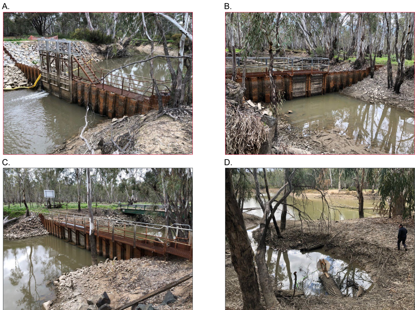
Figure 3: A) Tumudgerry Creek Offtake Regulator, B) Reed Bed Creek Offtake Regulator, C) Niemur River Offtake Regulator, D) Moonyah Lagoon Inlet Pipe
